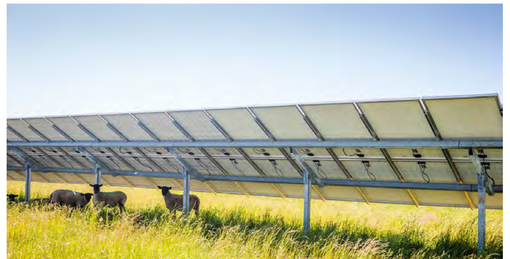
Tracker Solar Panels
